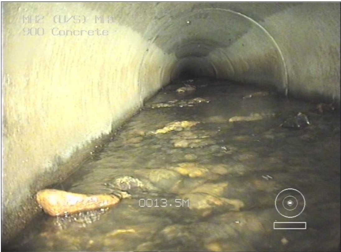
Photograph 7 – CCTV image of the culvert blockage
