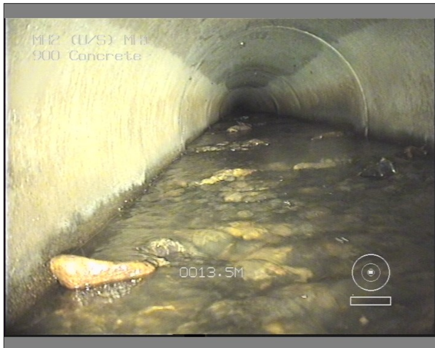
Photo: 1_1_10_A.JPG 13.5m, Settled deposits, coarse, 40% cross-sectional area loss, Start
