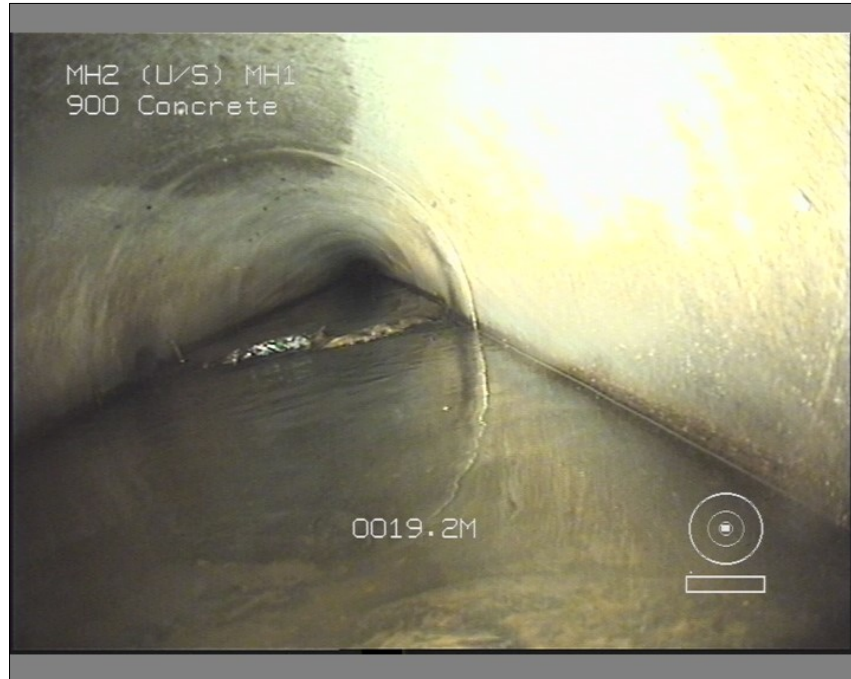
Photo: 1_1_12_A.JPG 19.2m, Settled deposits, coarse, 50% cross-sectional area loss, Start
