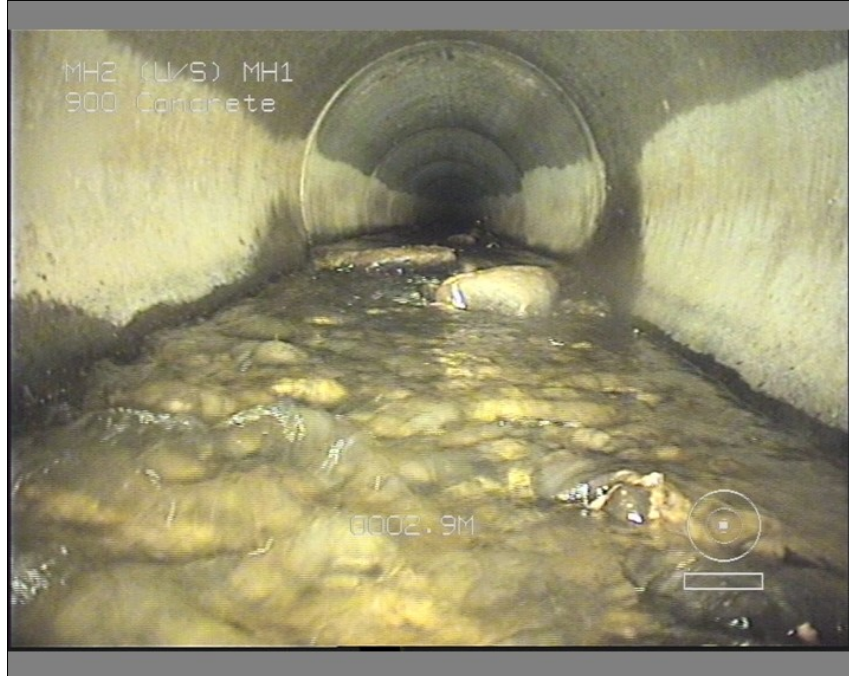
Photo: 1_1_5_A.JPG 2.9m, Settled deposits, coarse, 30% cross-sectional area loss
