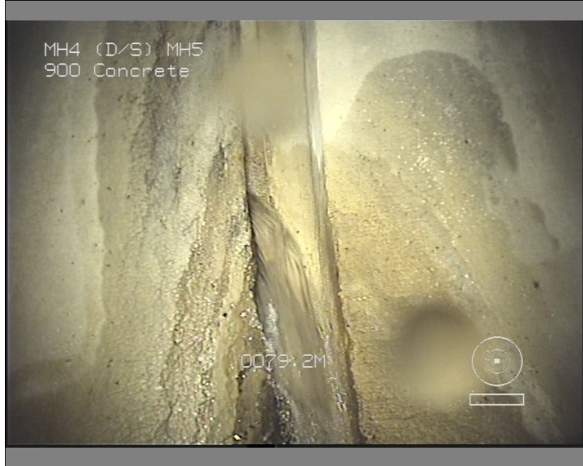
Photo: 5_5_24_A.JPG 79.2m, Infiltration, gushing at joint, from 7 to 10 o'clock
