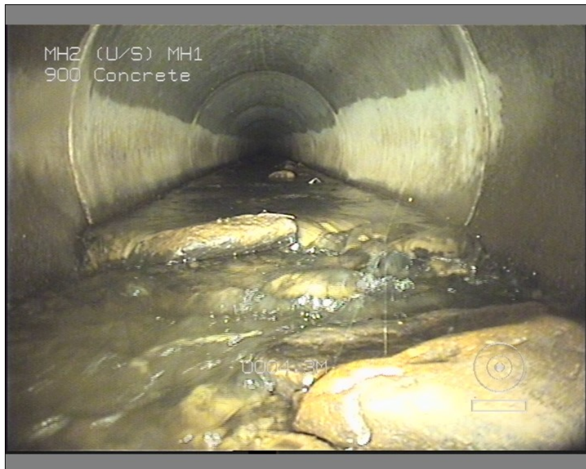
Photo: 1_1_6_A.JPG 4.3m, Other obstacles, brick or masonry in invert, from 5 to 8 o'clock, 30% cross-sectional area loss
