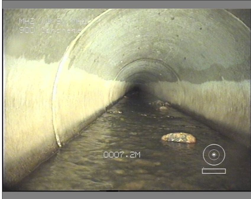
Photo: 1_1_7_A.JPG 7.2m, Settled deposits, coarse, 30% cross-sectional area loss, Start
